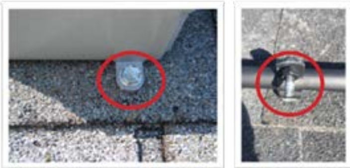
Photo 6: Roof penetrations and anchors not flashed: International Building Code 1503.2, International Residential Code 903.2.
