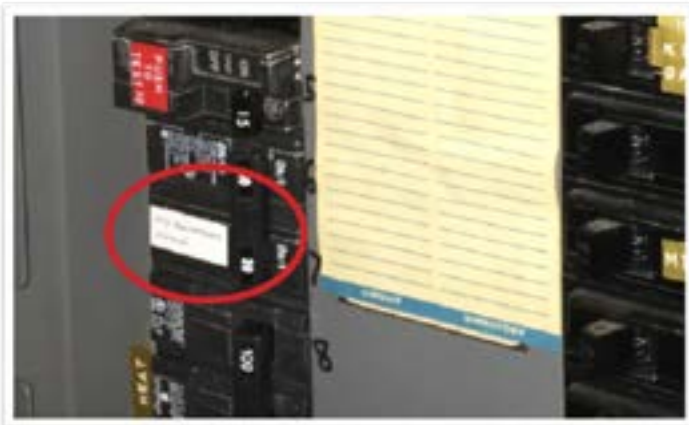
Photo 3: Working clearance not maintained: NEC 110.26
